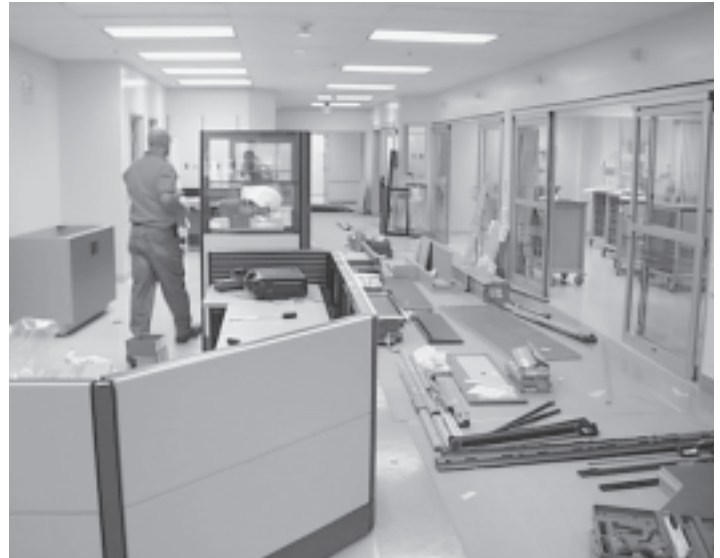
Construction workers scurry to finish the new Emergency Room at the Yukon-Kuskokwim Delta Regional Hospital.
