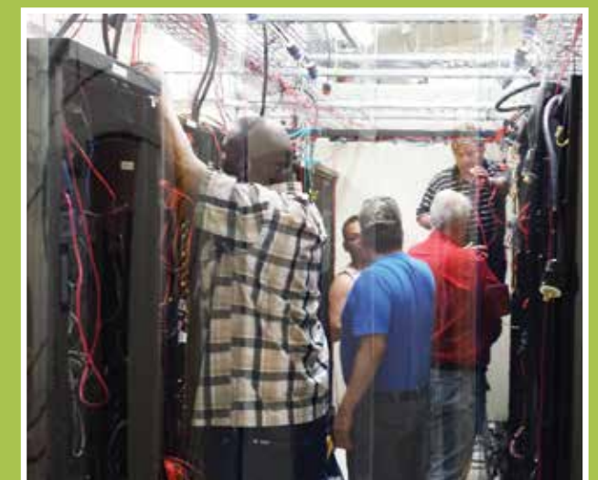
Technology Department staff spent a Saturday sorting a spaghetti bowl of wiring to reconfigure the company's vital cyber infrastructure.
